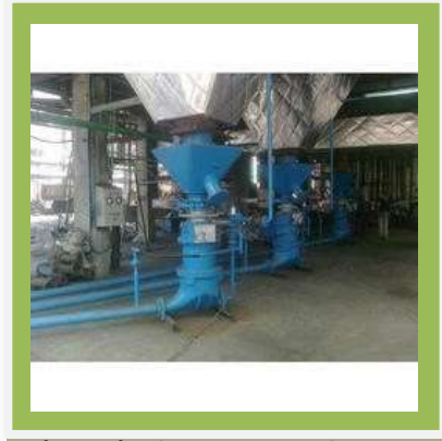
Fly Ash Conveying System
