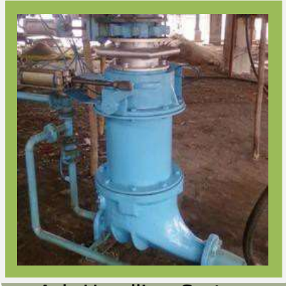
Ash Handling System
